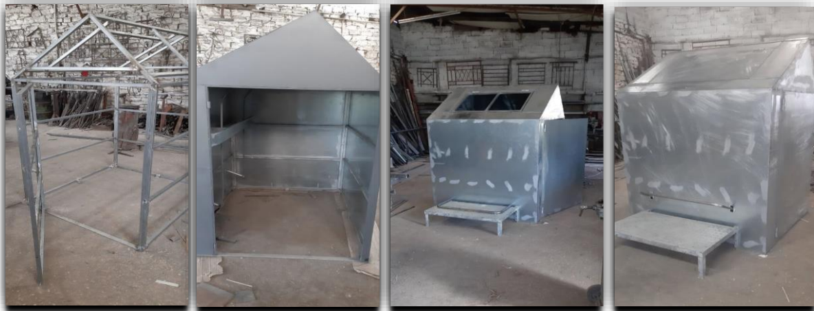
Figures 1-4. Photos of the construction process of the meta shell garbage bins
